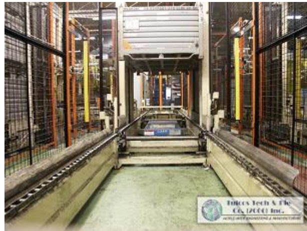
Conveyor line for material, containers handling, circulate U shape line, Central Stamping, Windsor
